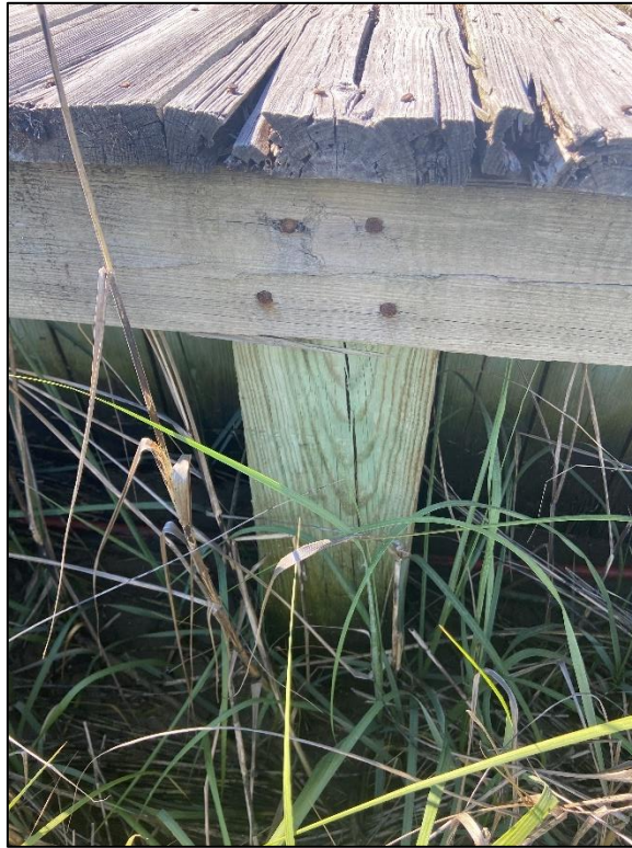
Figure 3.16. Connection with Four Rusted Nails
