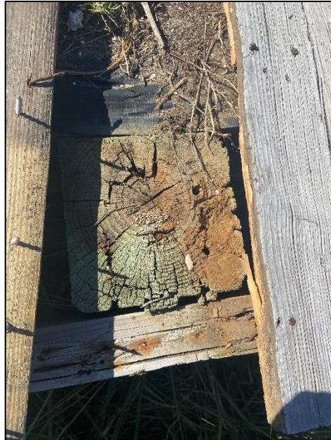
Figure 3.12. Deterioration in Top of Pile
