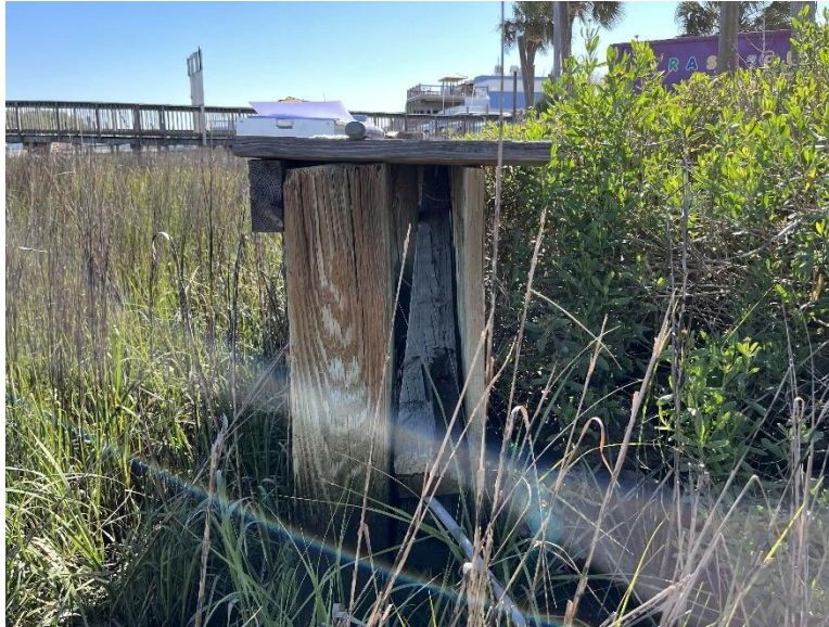
Figure 3.2. Collapsed Top Waler at West End of Bulkhead
