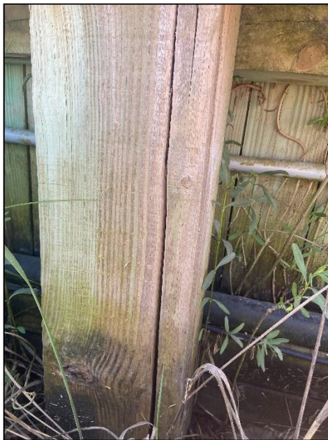
Figure 3.11. Longitudinal Split in Pile
