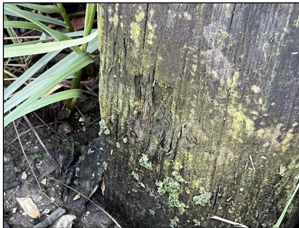
Figure 3.7. 8x8 Pile with Visible Deterioration Near Base at Mudline
