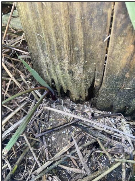
Figure 3.9. Rotten Pile at Base at Mudline
