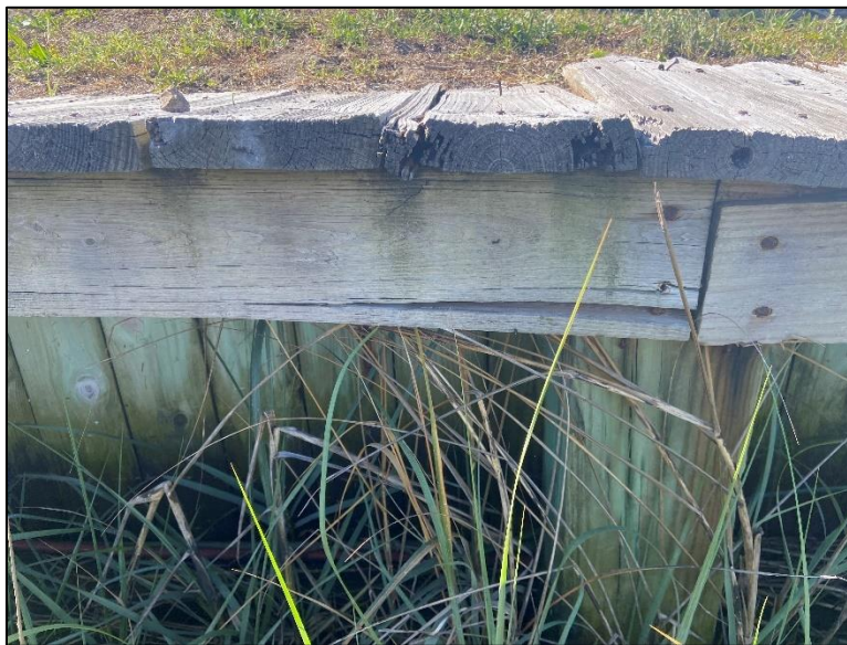
Figure 3.15. Connection with Two Rusted Nails
