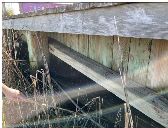
Figure 3.1. Collapsed Top Waler at West End of Bulkhead
