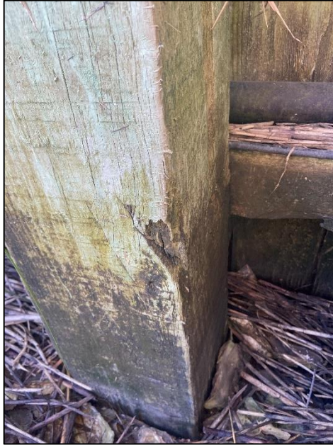
Figure 3.10. Minor Deterioration on Corner of Pile
