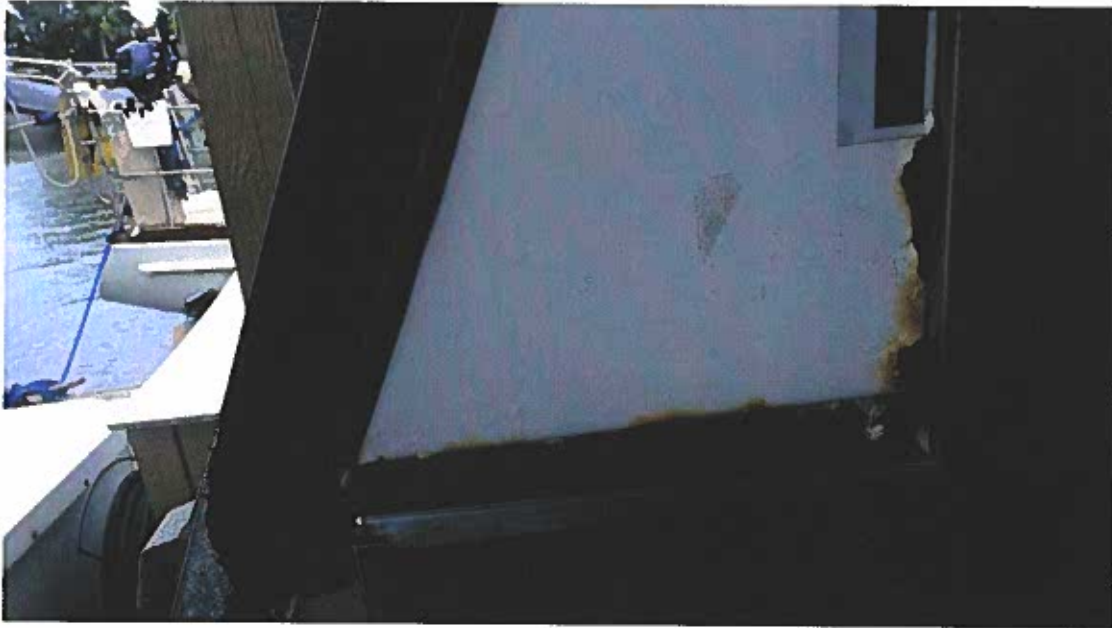
(Photo 19) Corroded fuel dispenser beyond repair.
