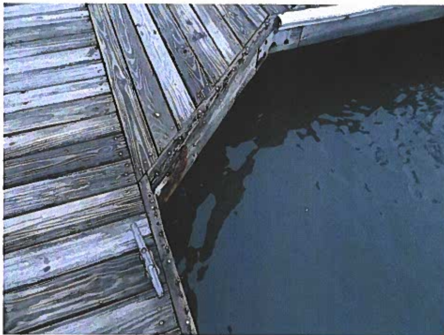
Bumper Strip Damage and Corroded Connection Hardware
