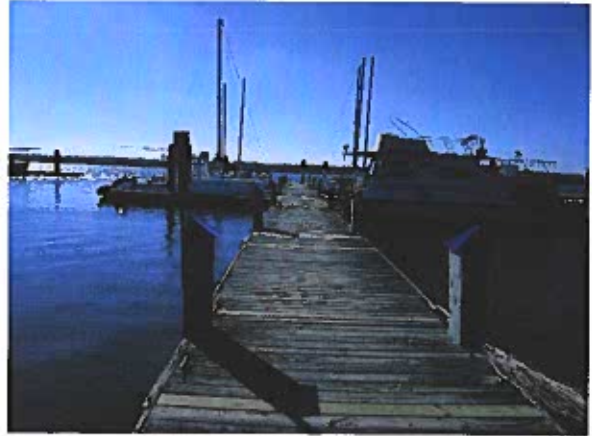
Typical Dock Conditions at Dolphin Cove Marina
