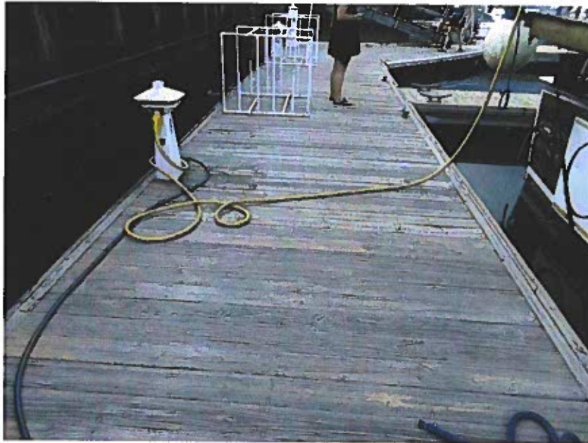
Power Cables Routed Across Main Walkway
