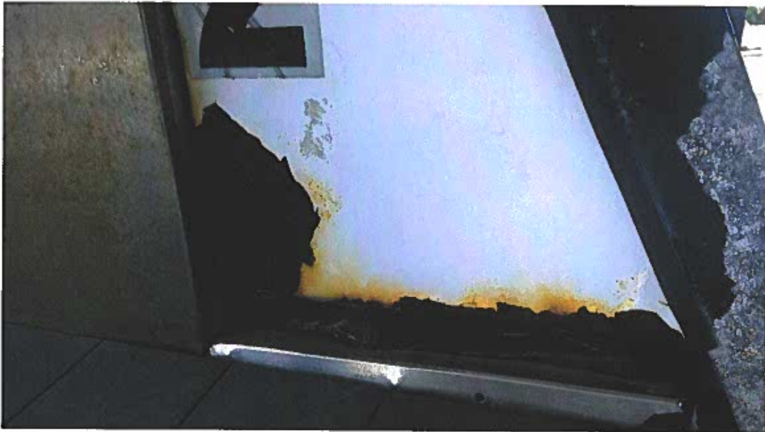
(Photo 20) Corroded fuel dispenser beyond repair.
