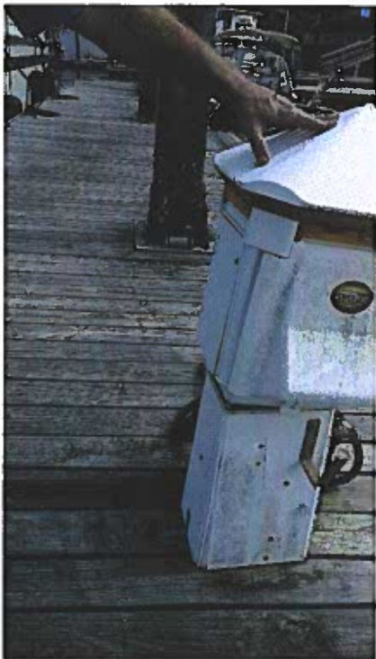
(Photo 2) Dock mounted pedestal missing fasteners and not mounted to dock.
