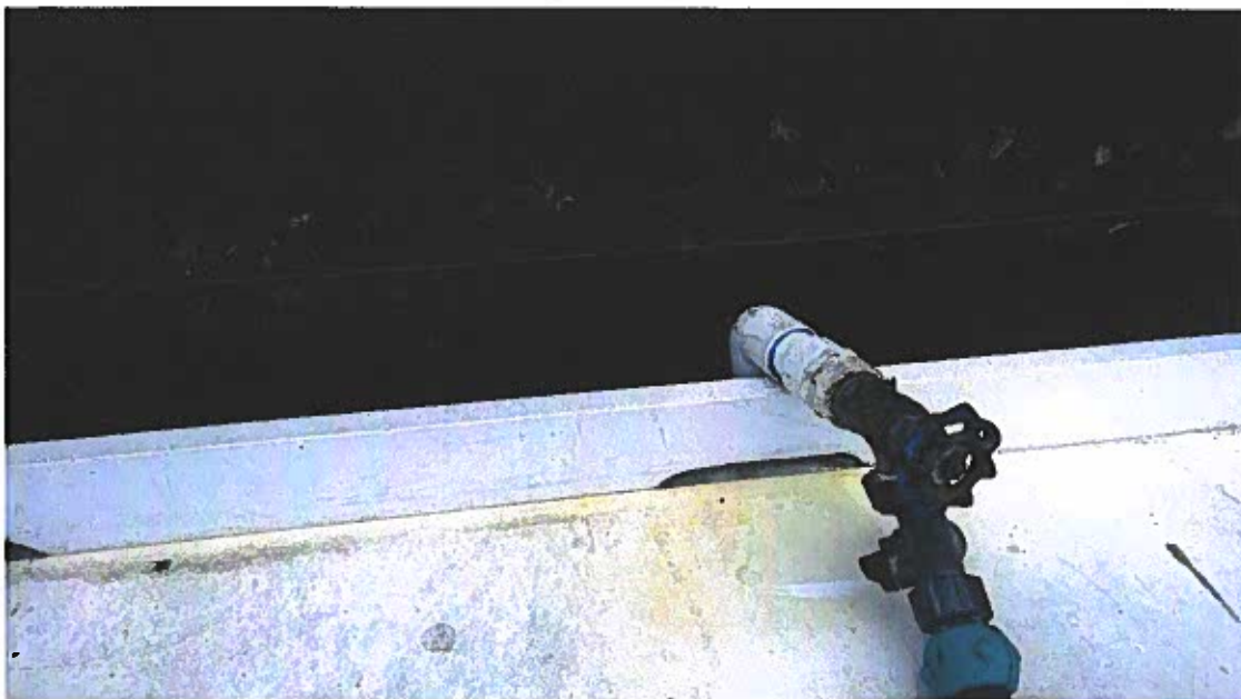
(Photo 15) None of the hose bibs are freeze protected nor are there any vacuum breakers on the hose bibs.
