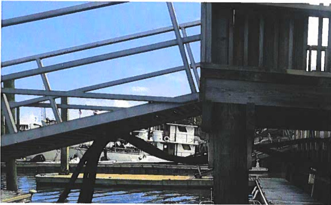
(Photo 6) The cabling to the marina is not properly supported.
