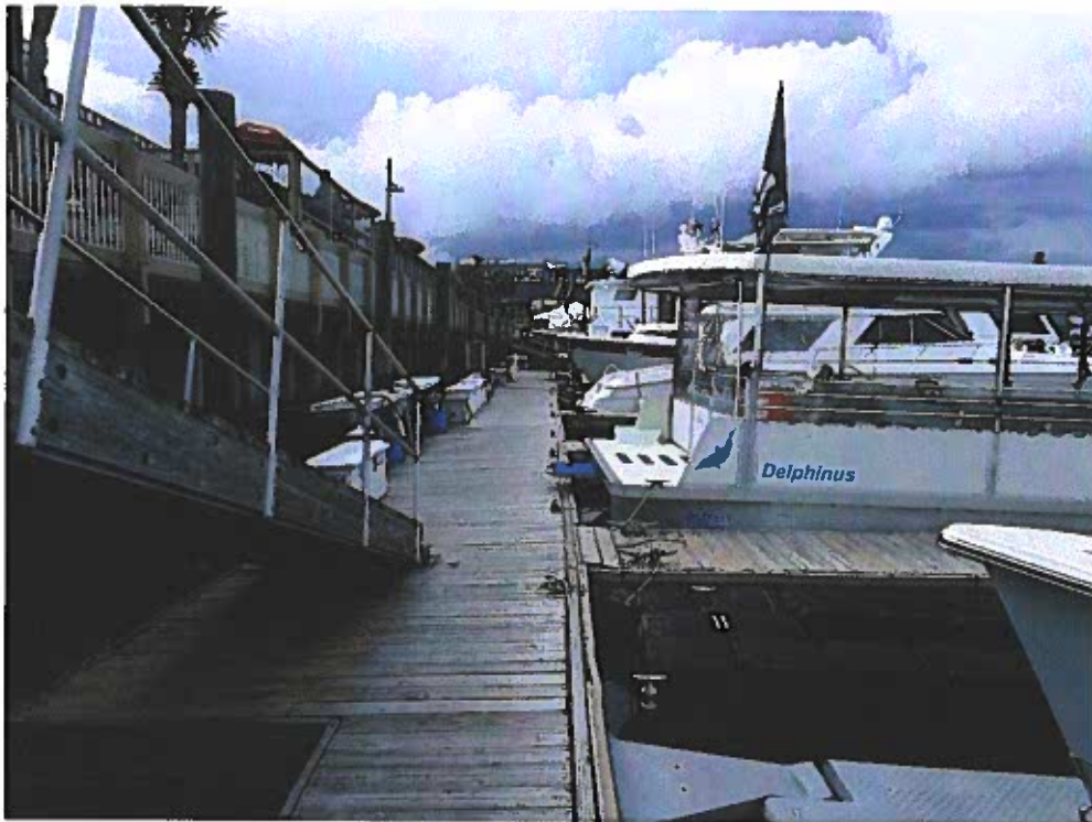
Shore-Parallel Main Walkway (Note: substantial landward listing)
