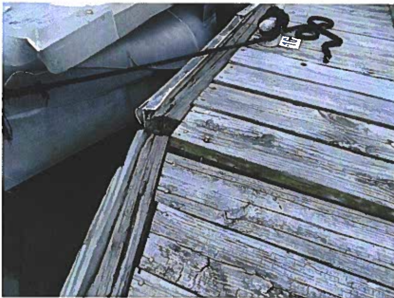
Framing Failure at Inflection Point
