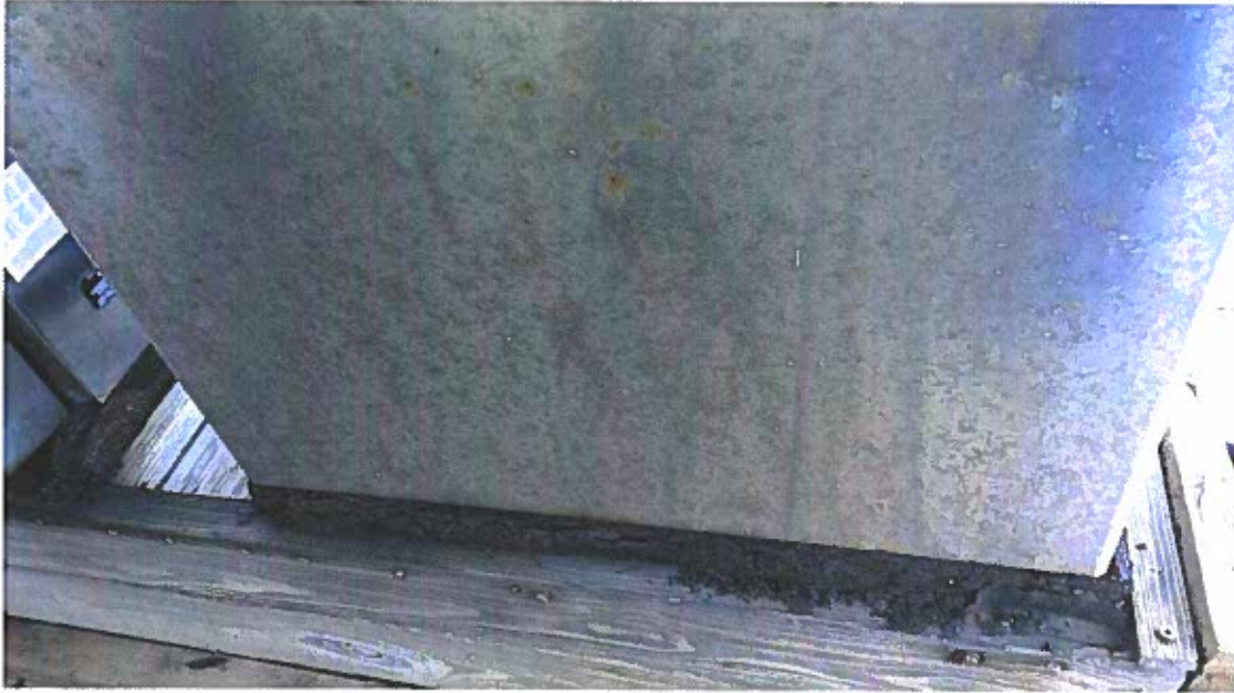
(Photo 21) Corroded fuel dispenser beyond repair.
