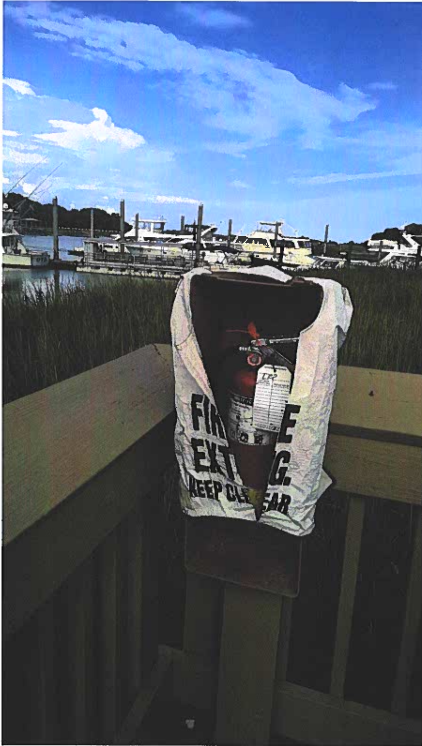
(Photo 18) Damaged fire extinguisher cover.
