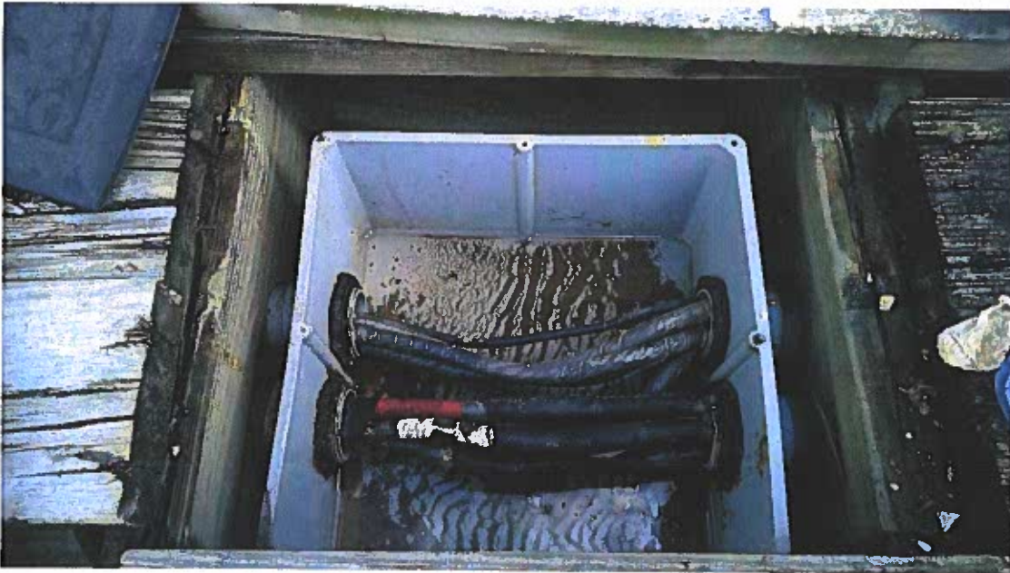
(Photo 4) There are junction and pull boxes that are not sealed from the salt water.
