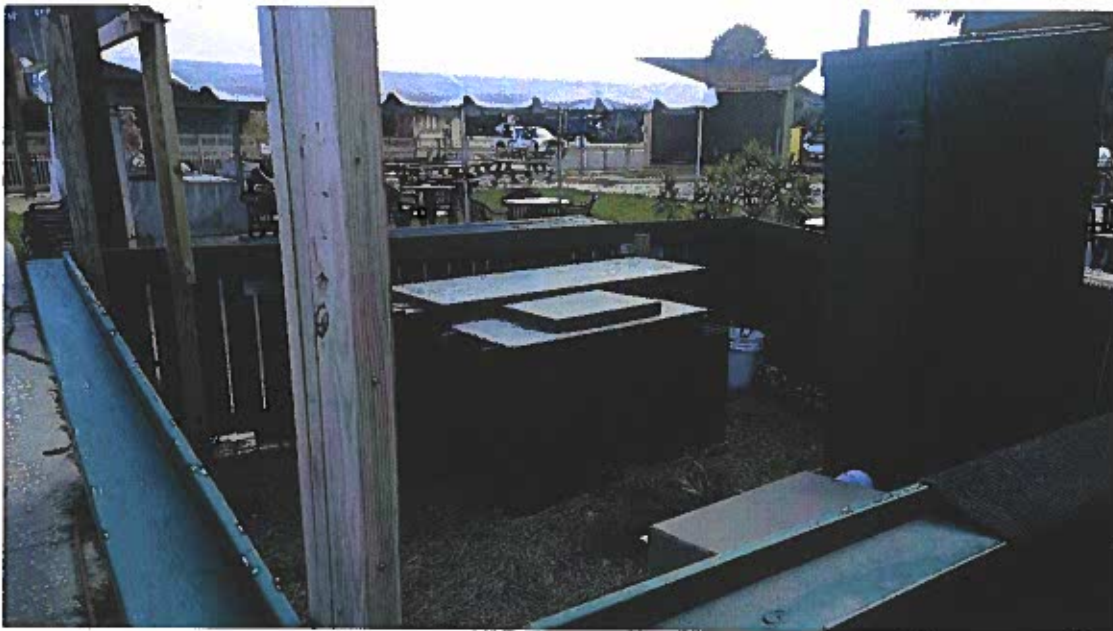
(Photo 8) The transformers are not level and the electrical panel does not have code required clearance.
