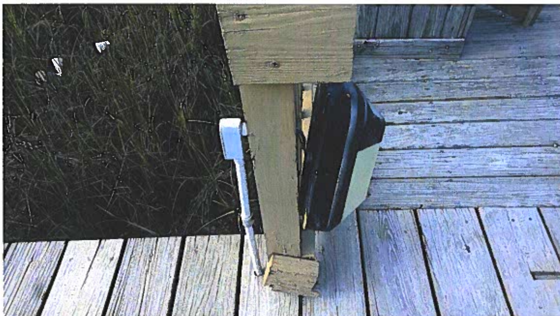
(Photo 11) Broken light fixture.
