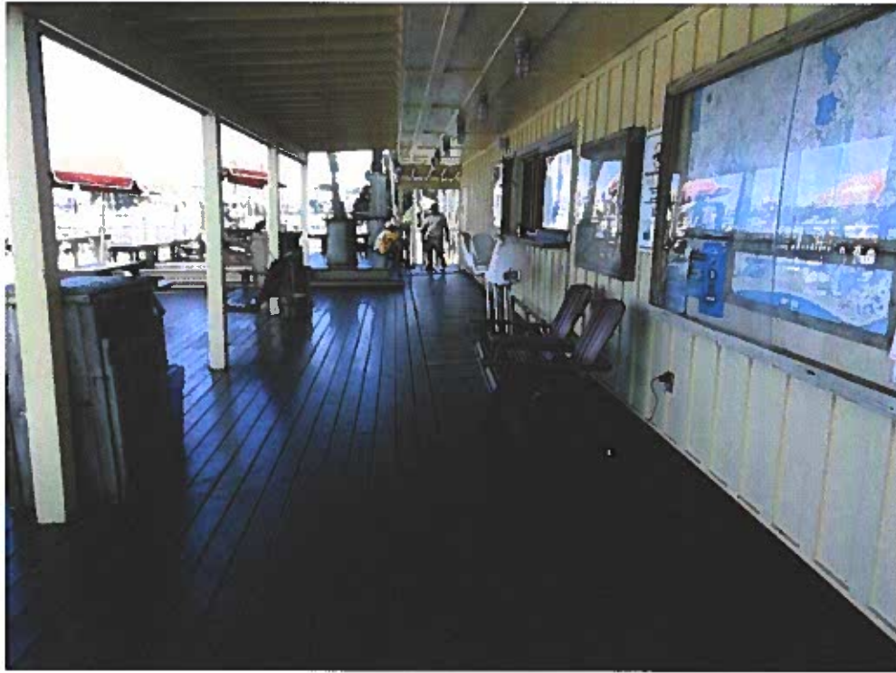
Marina Store – Rear Patio (Note: Walking surface slope away from building)
