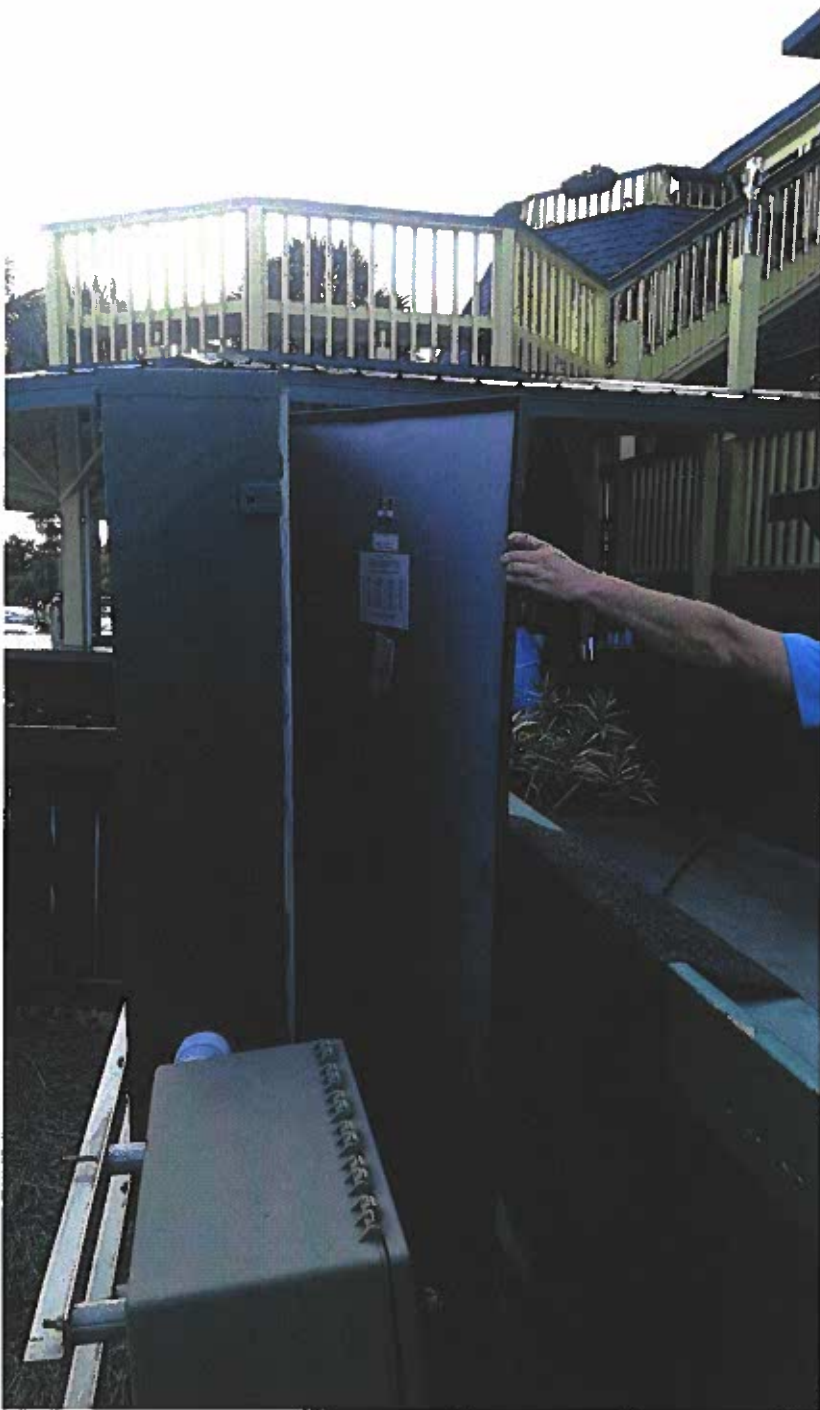
(Photo 9) The door to the panel is not able to open due to a fence and does not have code required clearances.
