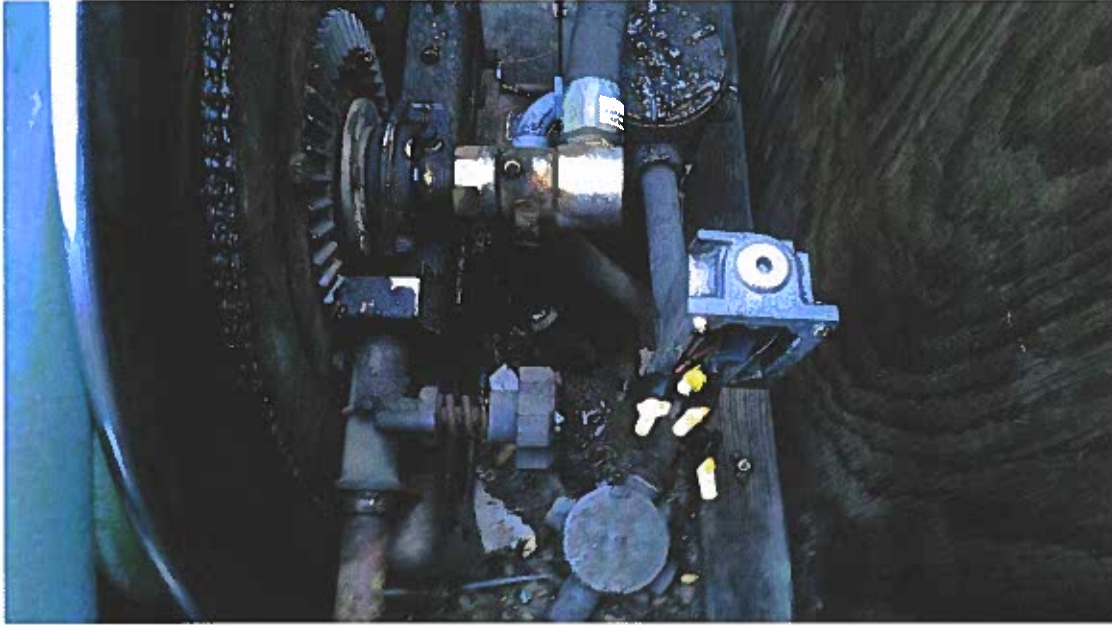
(Photo 12) Improperly sealed junction within 25 feet of fuel pumps needs explosion proof enclosure.
