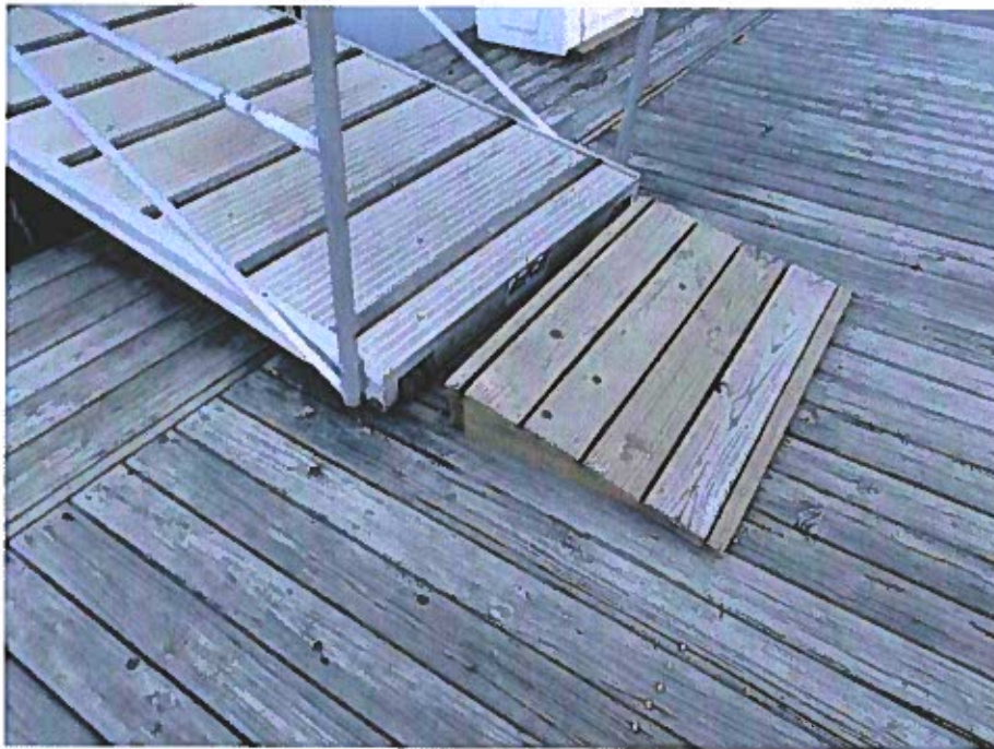
Gangway Landing "Wedge"
