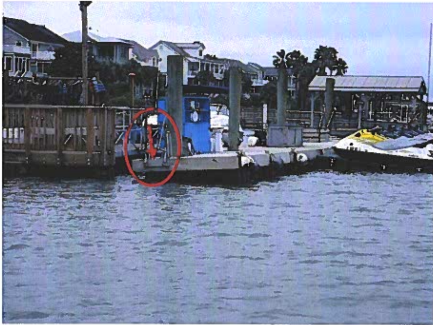
Severe Dock Listing
