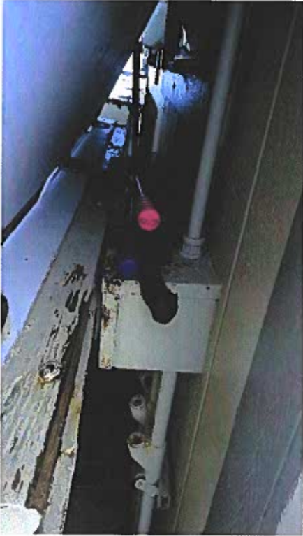
(Photo 3) Junction box rusted and in a wet location.
