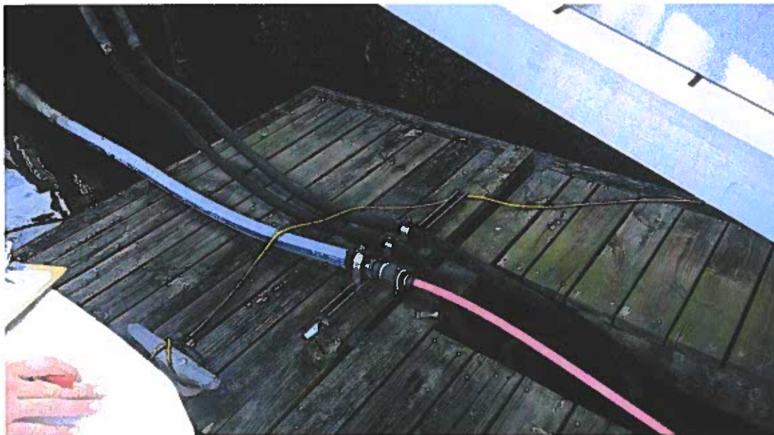
(Photo 13) The piping not properly supported and is subject to U.V. degradation.
