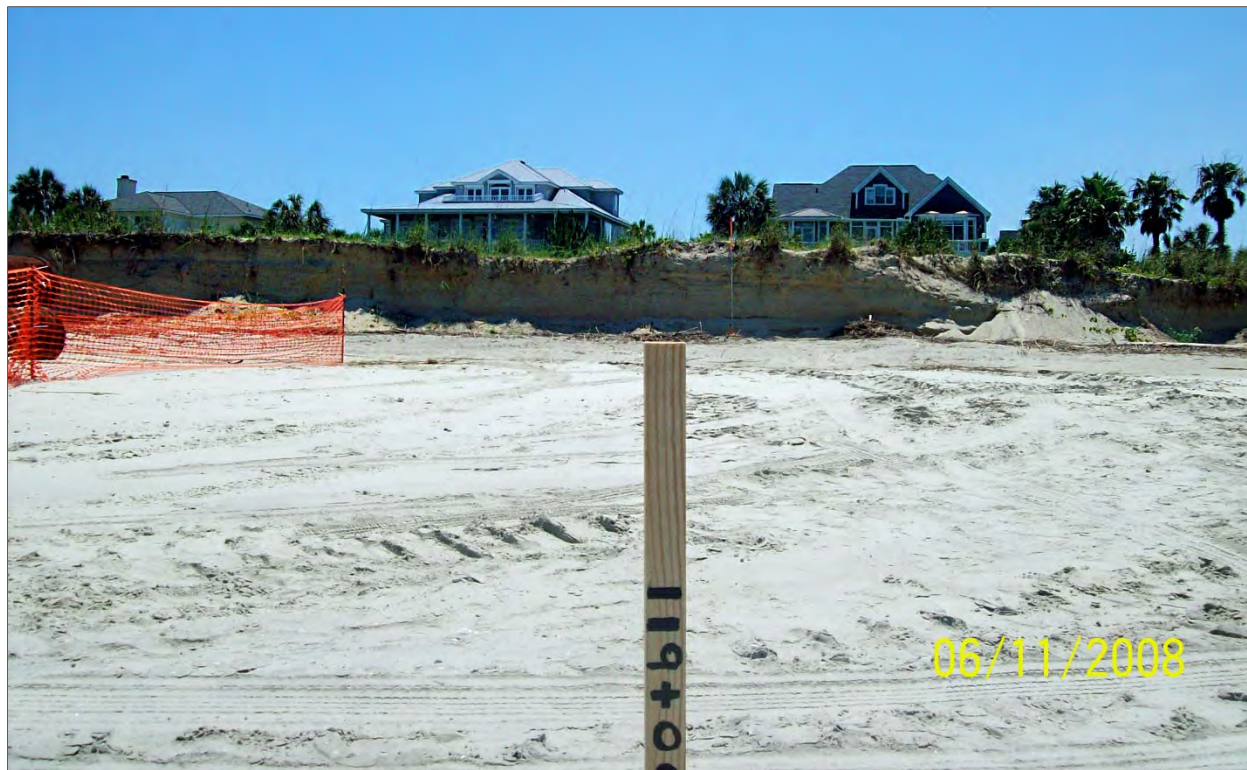
FIGURE 4.5. In 2008, a significant erosional escarpment was documented along most of Reach 7 seaward of the 17 th tee box of the Links Course.
