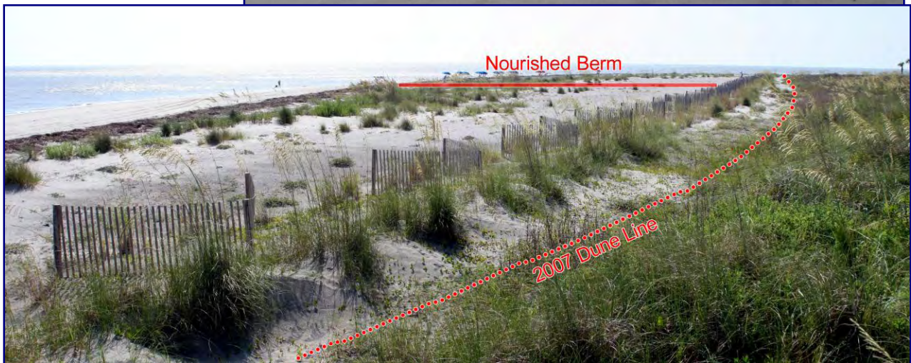
FIGURE 3.6. [UPPER] View looking south from station 332+00 in July 2013; the sand visible in this image has accreted since nourishment. [MIDDLE] Northwest view in July 2013 from station 344+00 ~400 ft seaward of the groin. A small scarp is visible; however, a dry berm separates the high waterline from the dune. [LOWER] View seaward of the nourished area of Reach 7 in July 2012. Vegetation has become well established seaward of the sand fencing. The pre-project dune line (red dotted line) is the dense vegetation ~25 ft to the right of the fencing in the image. [Photos by D Giles and S Traynum]
