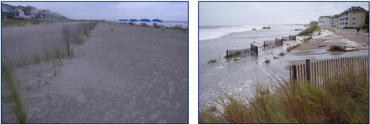
FIGURE 3.52. [LEFT] Sand fencing in Reach 5 in June 2011. There is less dune growth in this area than in Reach 6. [RIGHT] Sand fencing and vegetation in Reach 6 from Ocean Club in August 2011 during Hurricane Irene . The +6-ft NAVD berm was overtopped; however, only the dune near the Ocean Club boardwalk showed any damage. The +8-ft NAVD storm berm was not overtopped.
