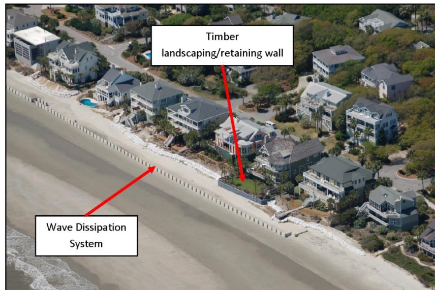
Figure 22. April 5, 2016 photo of Wave Dissipation System installation at Beachwood East (same area as shown in Figure 17). WDS ties into rock revetment at west end, see Figure 21. A timber retaining/landscaping wall is also shown.
