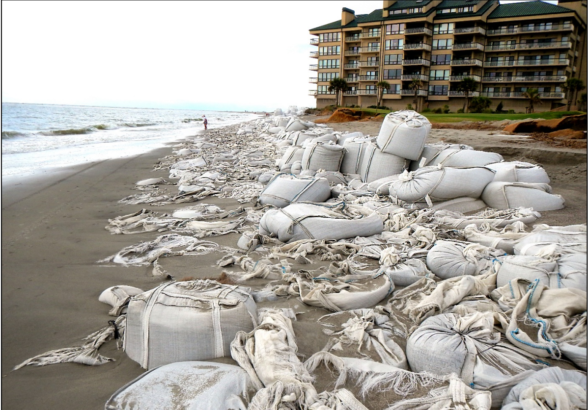
PHOTO 21. Looking south at the Ocean Club Villas in September 2014 during sandbag installation.
