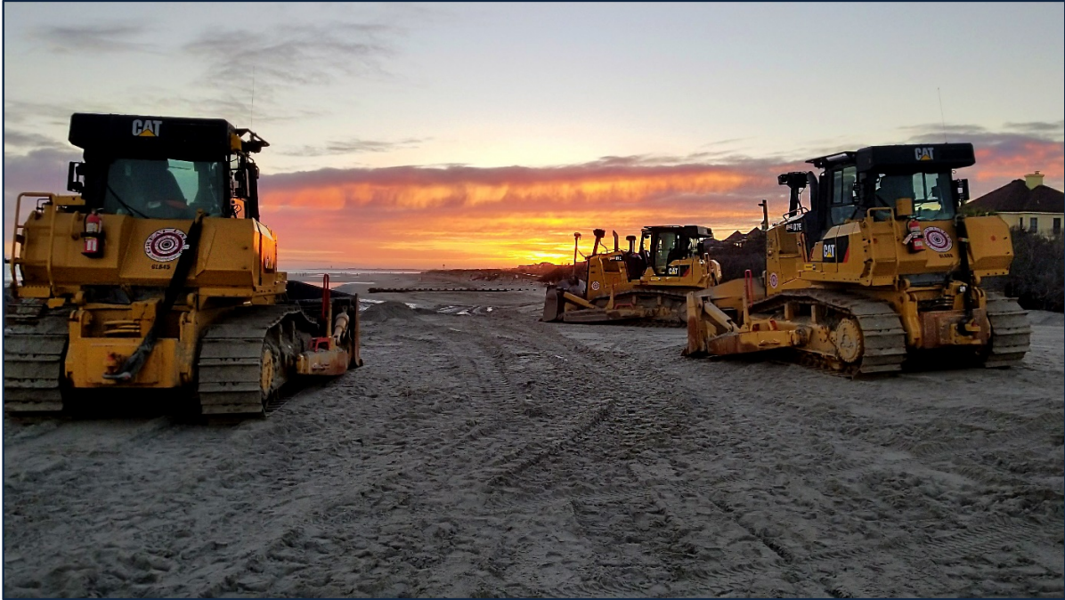
PHOTO 11. Bulldozers on standby ready to grade near the south end of Reach 1. [Image taken 23 February 2018]
