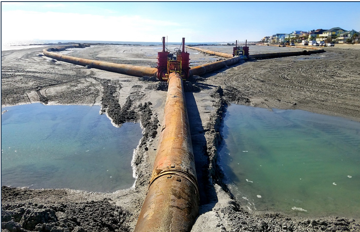
PHOTO 6. Three discharge points were used in some sections of the beach to accommodate for the large berm specifications of the design.
