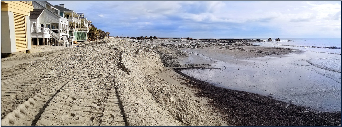
PHOTO 7. Pumping and beach grading operations underway on 22 January 2018 in front of Beachwood East.
