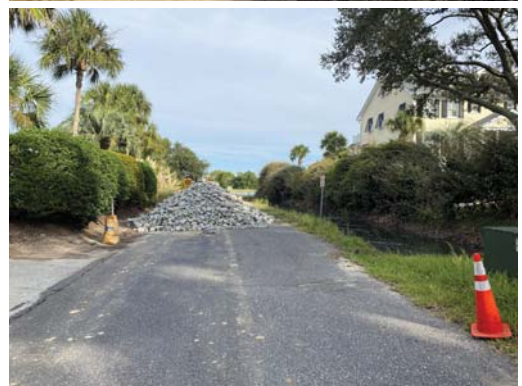
Check valve and earthen berm installation at 25th Avenue by SCDOT in October 2022.
